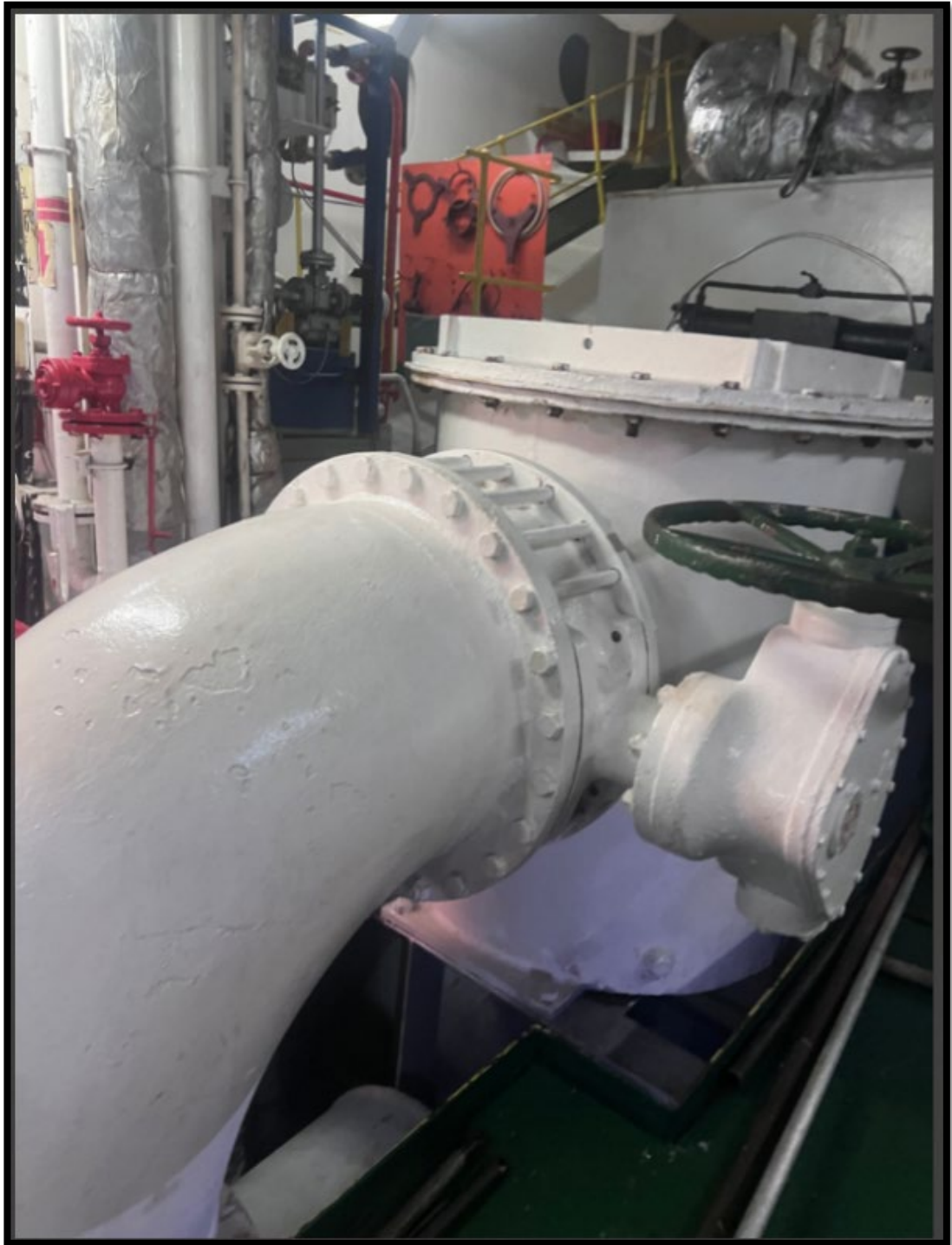
Figure 10 – The main seawater pipe from a sea chest filter
